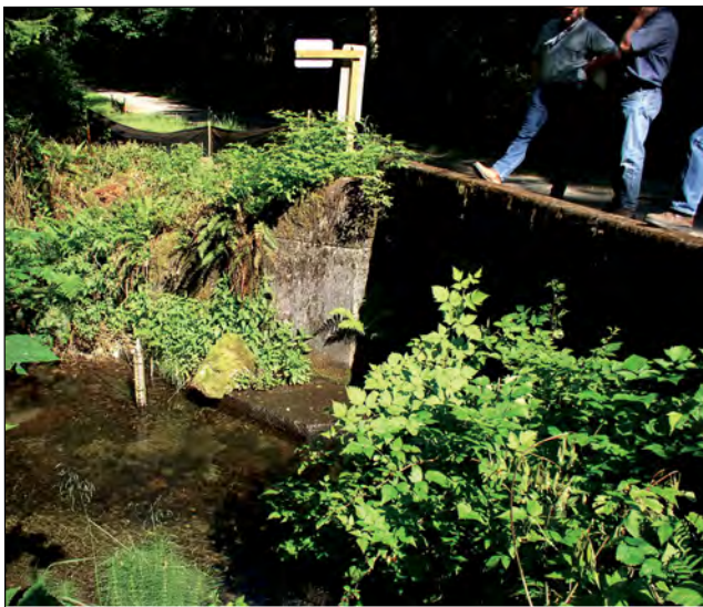
A turbidity sensor was installed in a tributary of the Cedar River watershed to monitor water quality conditions for Seattle, Washington.
