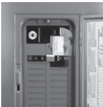
Generator Interlock Kit Installed
