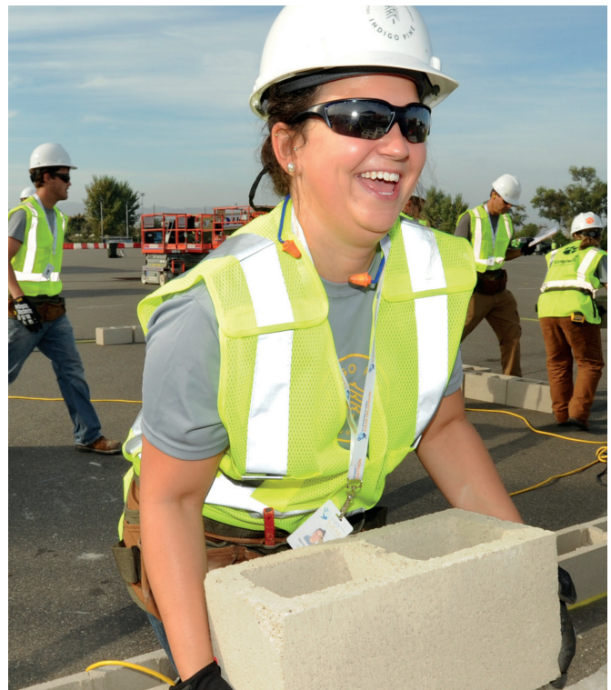
Melody Bazzle of Clemson University smiles as she and members of her team lay a foundation for their house at Solar Decathlon 2015 in Irvine, California. (Credit: Thomas Kelsey/U.S. Department of Energy Solar Decathlon)
