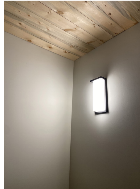
Figure 16: Electric lighting in the house
