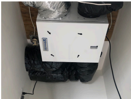
Figure 13: ERV on ceiling of mech room
