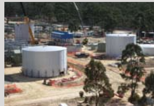
Water supply for mining
