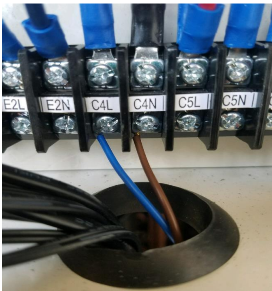
Pump power wires.
