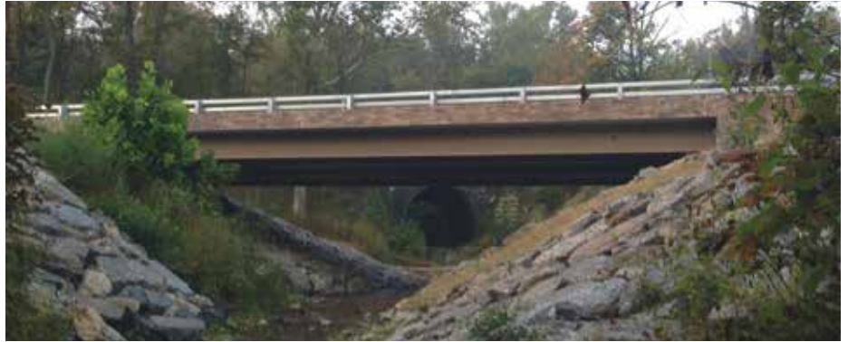
The new structure consists of three side-by-side, 23.7-m precast modules with Ductal® UHPC connections. Each module comprises two composite steel I-beams with a concrete deck slab. Additional elements were used to assemble the substructure. ABC methods made it possible for the bridge to be reopened to traffic in less than 7 days!
