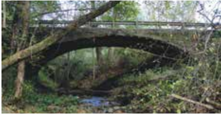
Fast replacement of a structurally deficient, single-span concrete bridge: State Route 288 Main Street Bridge in Wampum, Pennsylvania.
