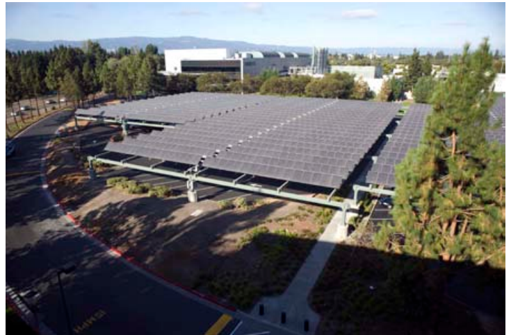
Applied Materials changed its parking lot to a power plant with what was, at the time, the largest corporate solar installation (2 MW) in Sunnyvale, California.
