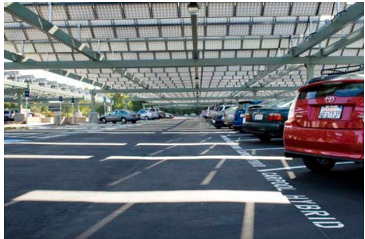
The parking lot solar plant provides shade for employee vehicles while generating substantial power.
