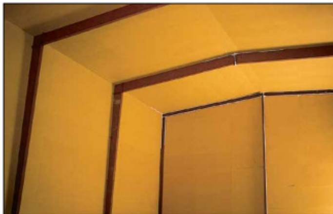
MDO panels are applied to the interior of a cold storage building.
