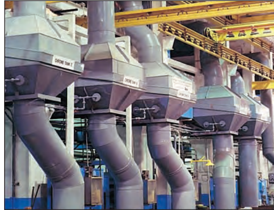
Harvel CPVC duct exhausts chromic acid fumes from plating operation
