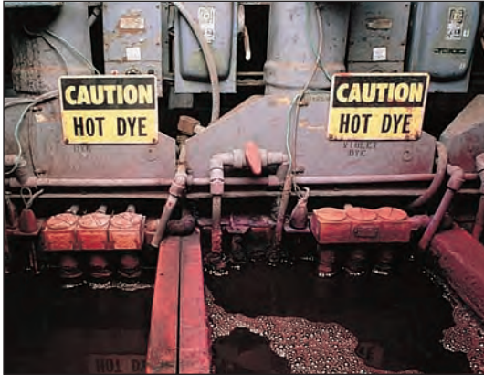
Schedule 80 CPVC piping transfers hot sulfuric acid dyes
