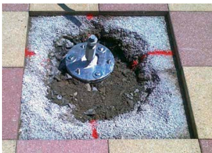
Spider Anchor VI with galvanised clamping plate at clinical clean construction site
