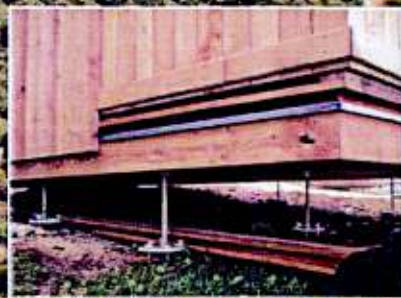
Foundation detail. The base frame of the building is supported via threaded rods on the solder sheeps anchors.
