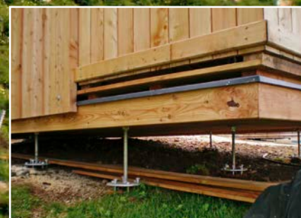
Foundation detail: The base frame of the building is supported via threaded rods on the spider-shaped anchors
