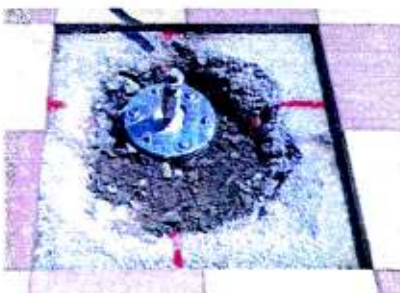
Spider Anchor VI with galvanised clamping plate at clinical clean construction site
