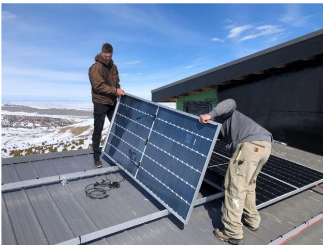
Figure 12. Rooftop Solar PV installation at the Wind River home
