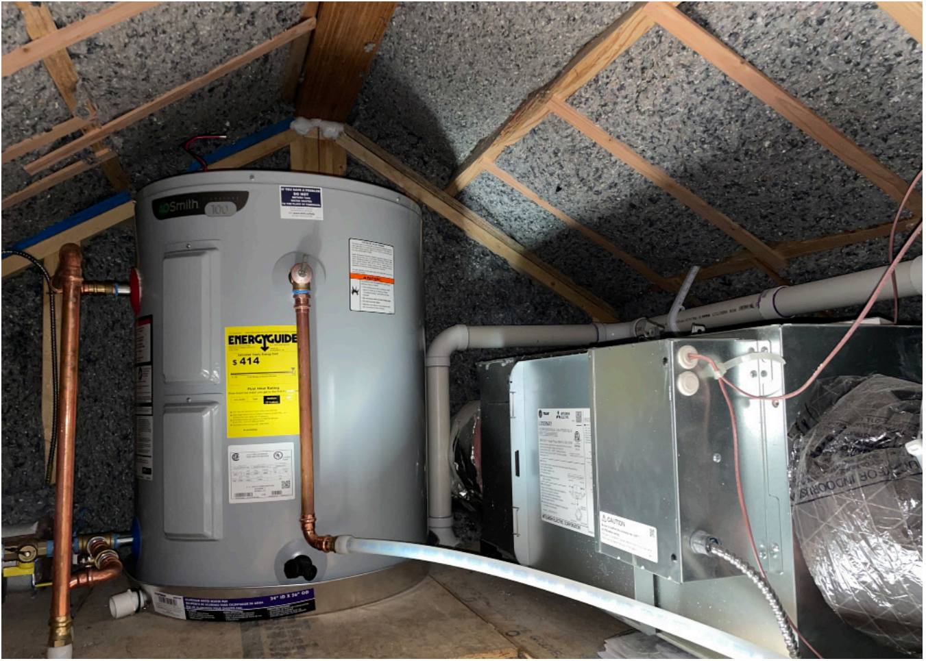
Haven Studio, photo of interior showing the mechanical loft.
