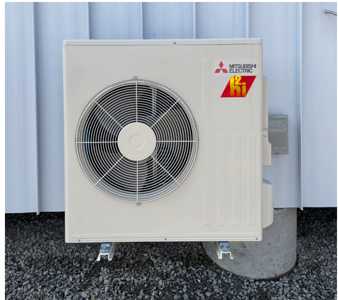
Haven Studio, mini split condenser unit attached to the standing seam north wall.
