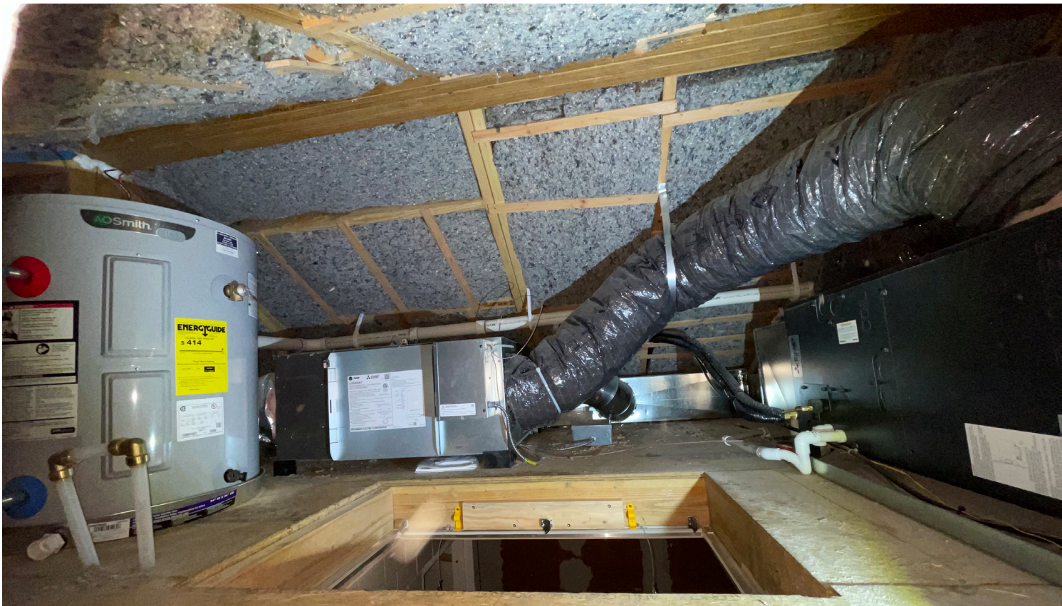
Haven Studio, inside the mechanical loft showing the hot water heater, ERV and fan coil unit for the mini split.
